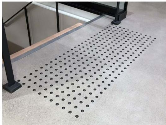
Figure 4.2 – Example use of Stainless-Steel Domes to Indicate Change in Floor Level
